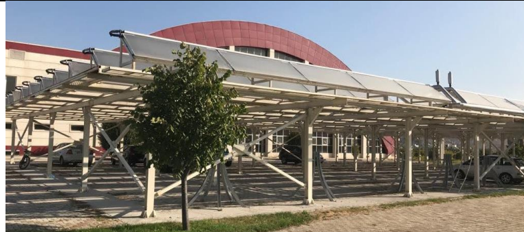
Solar absorption for heating the water used in school of medicine and swimming pool
